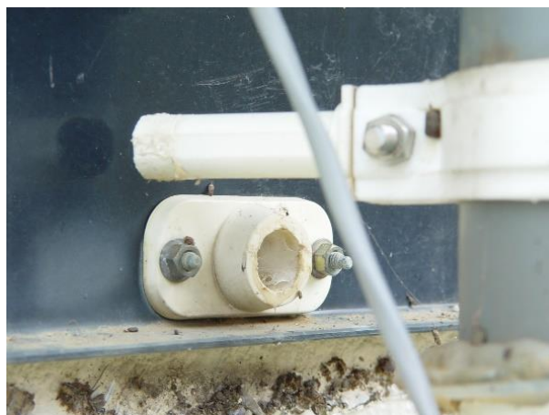
Picture 13. Failure of plastic pipe straps (not recommended).
