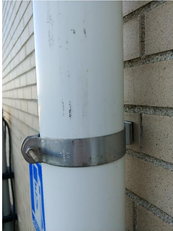
Picture 16. Electrical conduit strap (not recommended)
