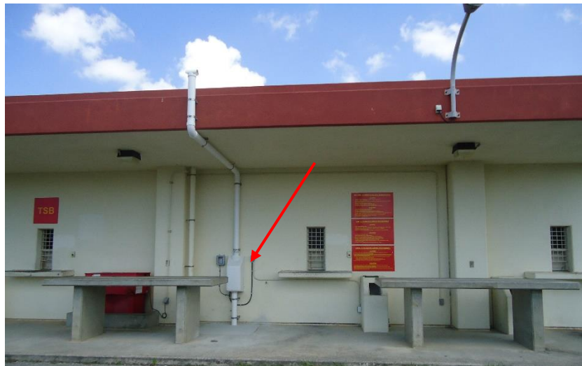
Picture 3. Typical single-story SSD installation.
