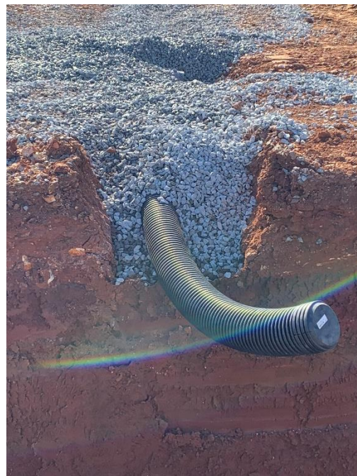
Picture 37. Buried perforated pipe.
