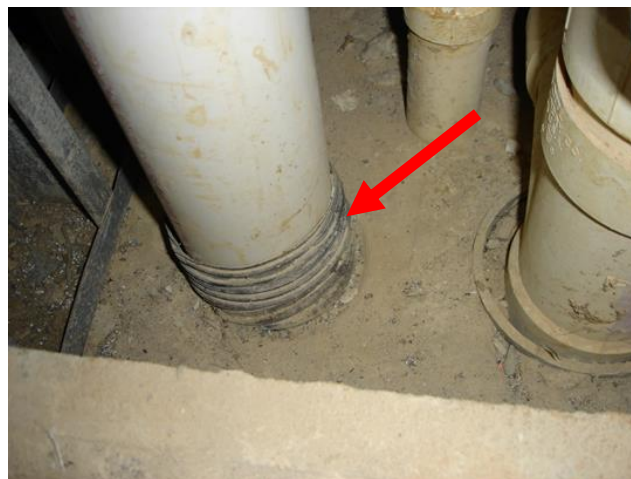
Picture 36. Example of a noncompliant RRNC system connection.
