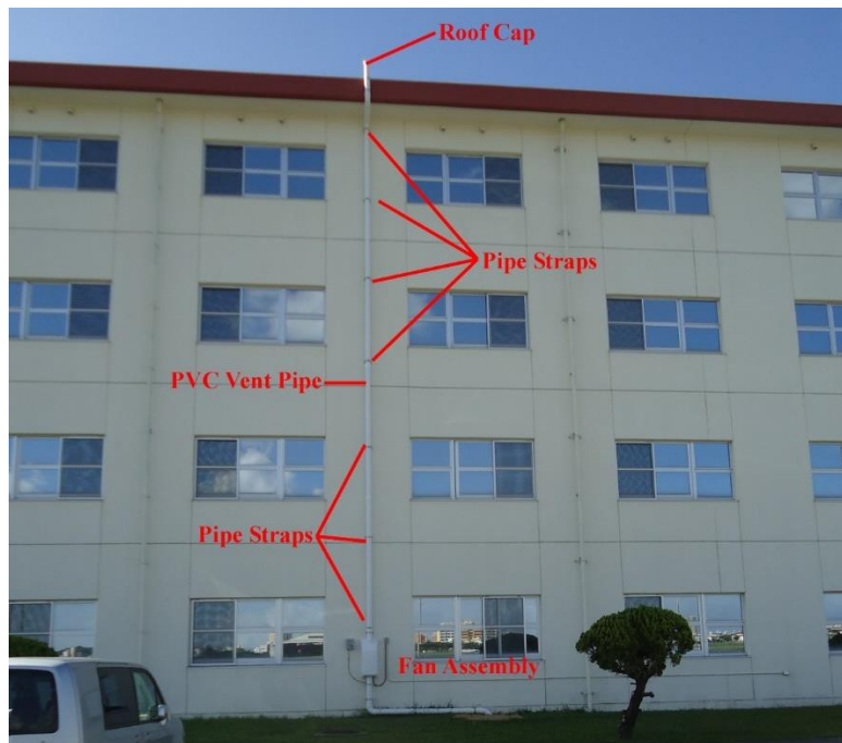
Picture 6. Typical pipe assembly for an SSD mitigation system.
