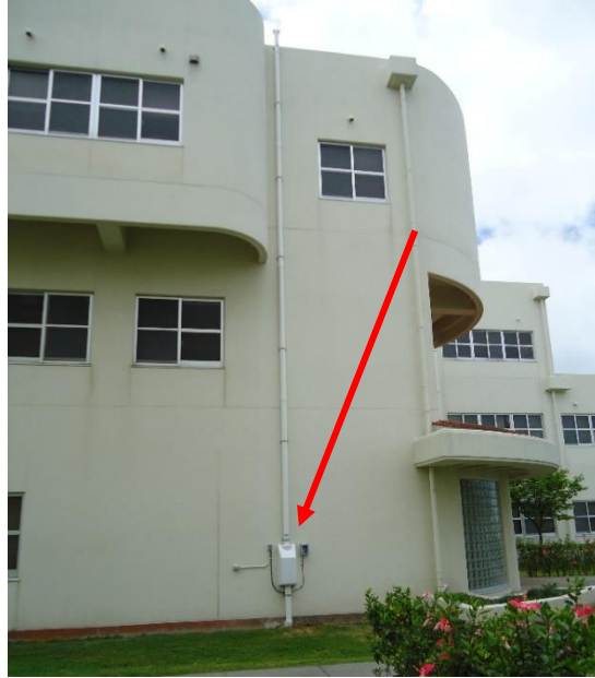
Picture 4. Typical two-story SSD installation.
