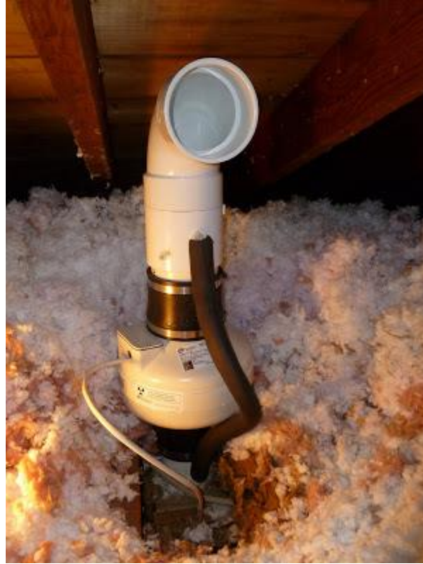
Picture 11. Attic discharge (not allowed).
