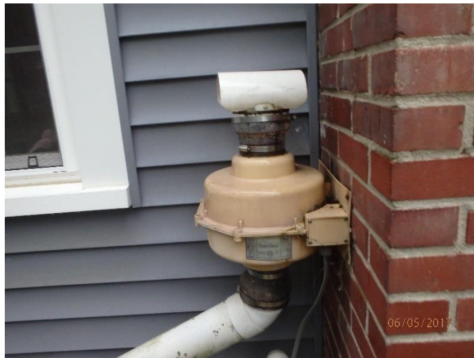
Picture 10. Radon exhaust near window (not allowed).
