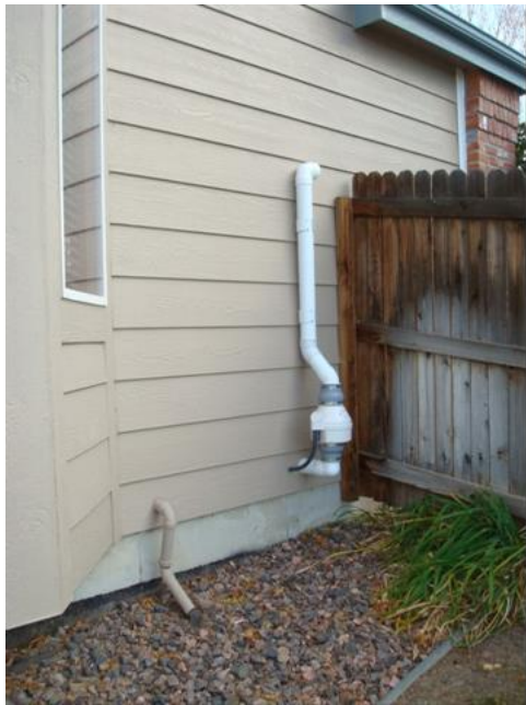
Picture 9. Side wall discharge (not allowed).
